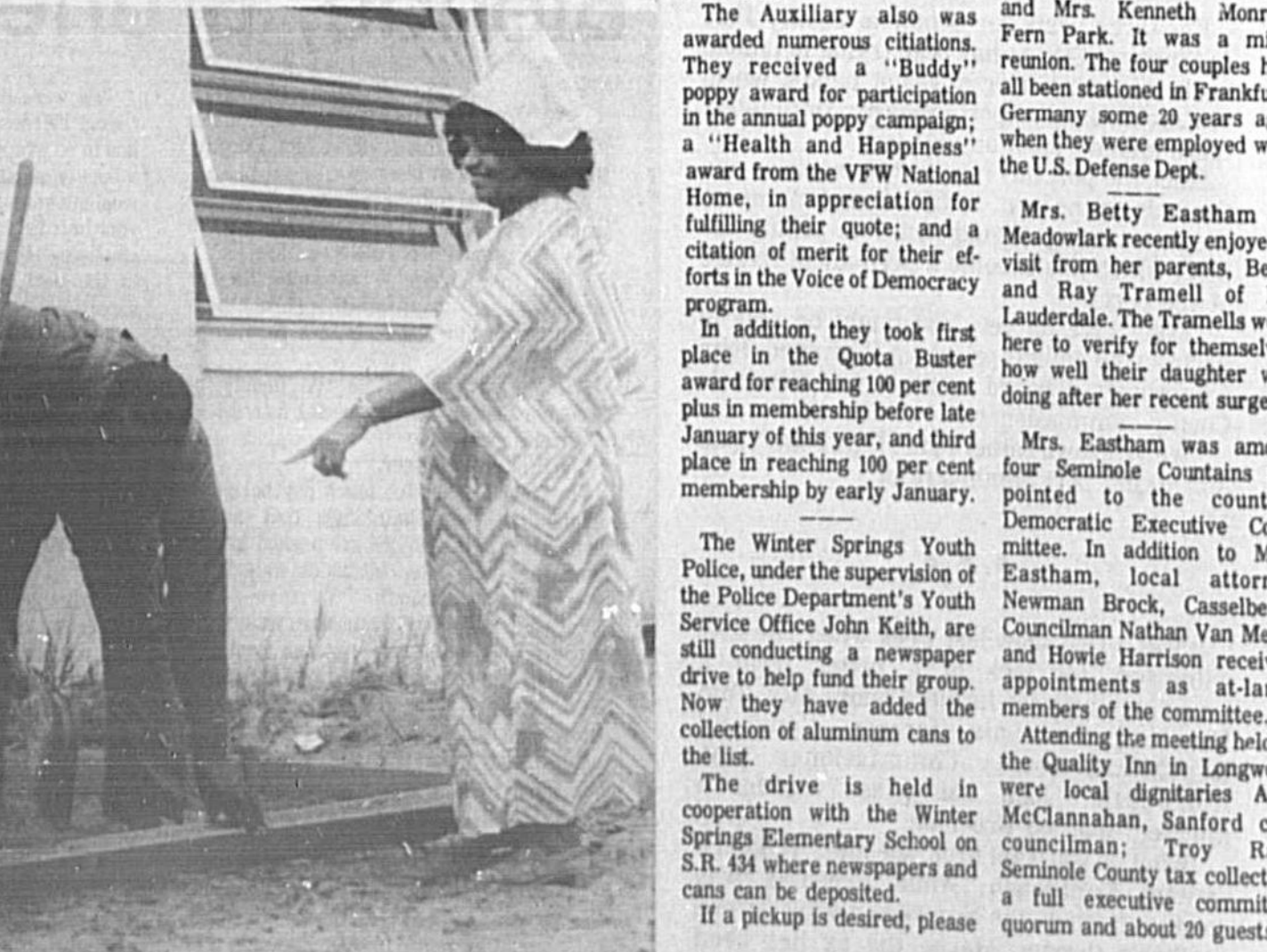
Mary Smith cracks the whip over volunteer workers (from left) J. W. McCudden, M.C. Anderson and Charlie Lyons as they lend a hand to get the foundation laid of the new patio being added to the Good Samaritan Home, Sanford. More volunteers, and additional funds are needed to complete the project.
