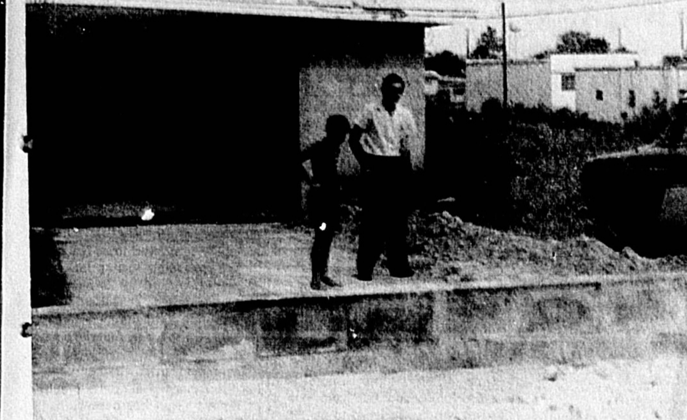
DIKING IN on Jewel Drive in Forest City, such as is being done here by M. H. McGaffigan and son, Andy, will not be necessary once the road is paved. Project was approved Tuesday by the County Commission. (Herald Photo)
