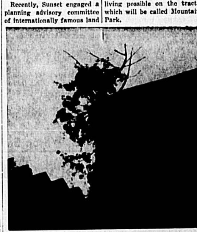
A TREE MAY have grown in Brooklyn, but in Sanford, a tree is growing from top of old Picot Hotel, corner of Commercial Street and Railroad Avenue. Trees roots eventually have taken the firm hold and gradually are dislodging bricks. Tree appears to be of camphor variety.
