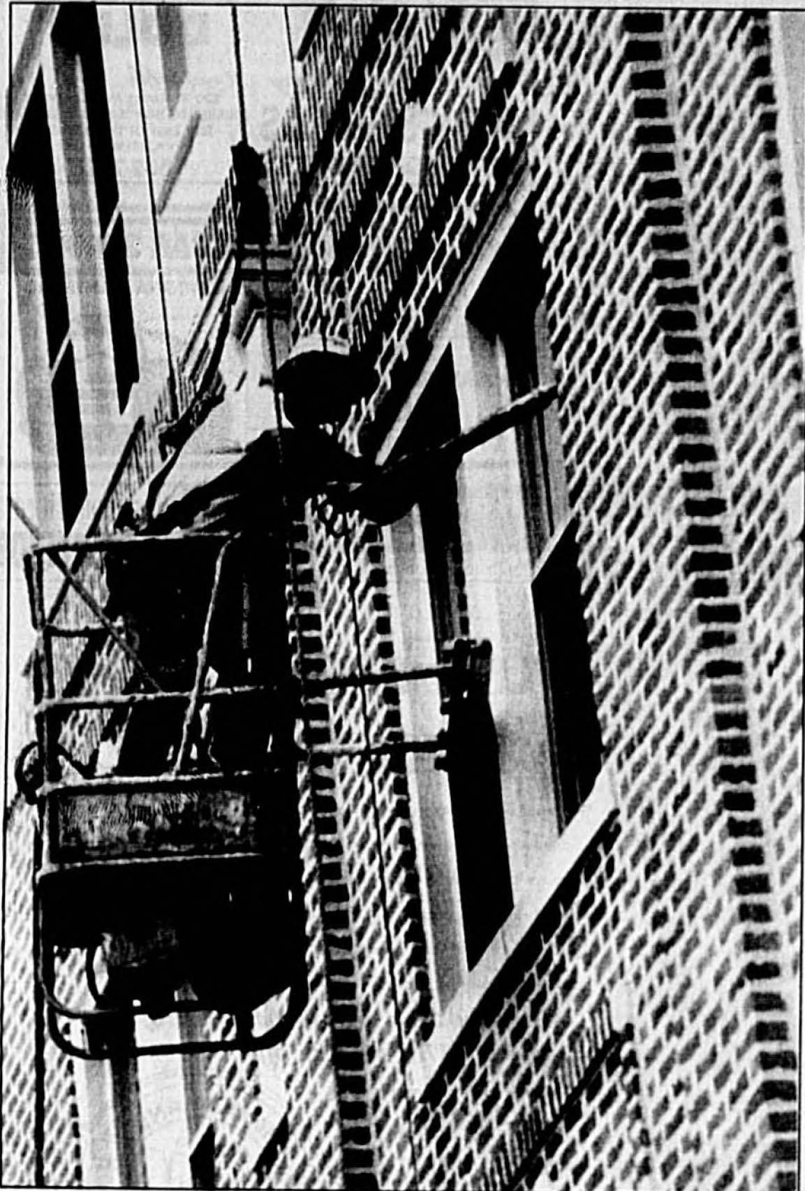
Tim Hoff, an employee with Moss Water Proofing and Painting Co. in Winter Park, leans out from his safe perch to apply caulk around a window at the State's Attorney's office, located at the corner of Park Avenue and First Street in downtown Sanford. Herald photo by Tommy Vincent
