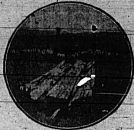
BROKEN WOODEN CULVERT.
