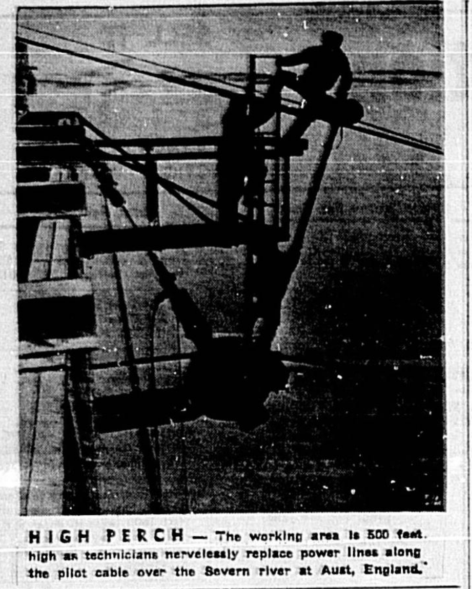
HIGH PERCH — The working area is 500 feet high as technicians nervously replace power lines along the pilot cable over the Severn river at Aust, England.
