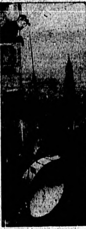
ONE OF THE FOUR giant beacons which will be installed atop the Empire State Building in New York is hoisted into position on the 80th floor. The new lights, which engineers say will be seen for a radius of 300 miles, will be 1,092 feet above the street. They are expected to be ready for Easter Sunday. (International)
