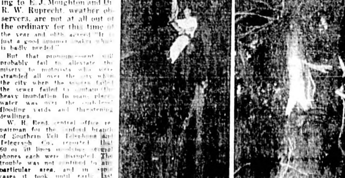
TELEPHONE TROUBLE—Charles Inghart, repairman for the Southern Bell Telephone and Telegraph Company, is shown in a pole at 14th St. and Laurel Ave., making repairs following the storm here Saturday. (Staff Photo)
