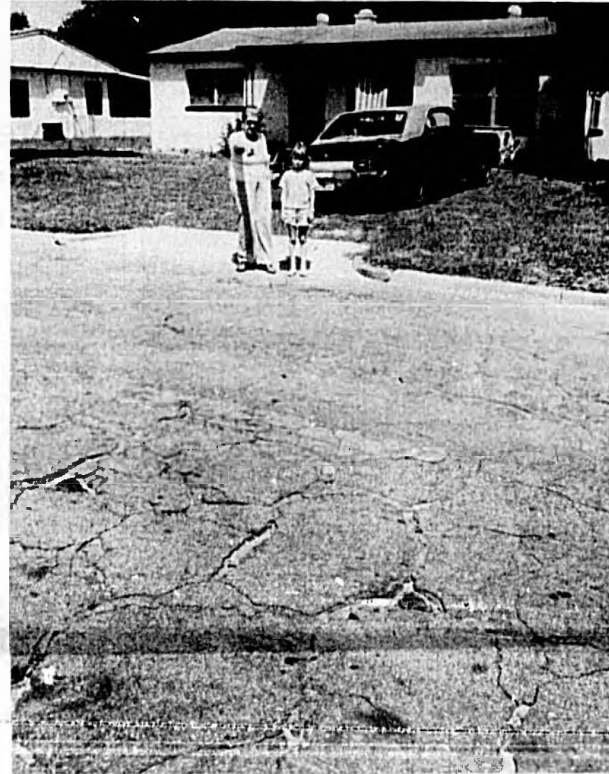
Ruth Bennett and granddaughter Julia Coffman show cracks in front Mrs. Bennett's home along East 4th Street in Sanford.
