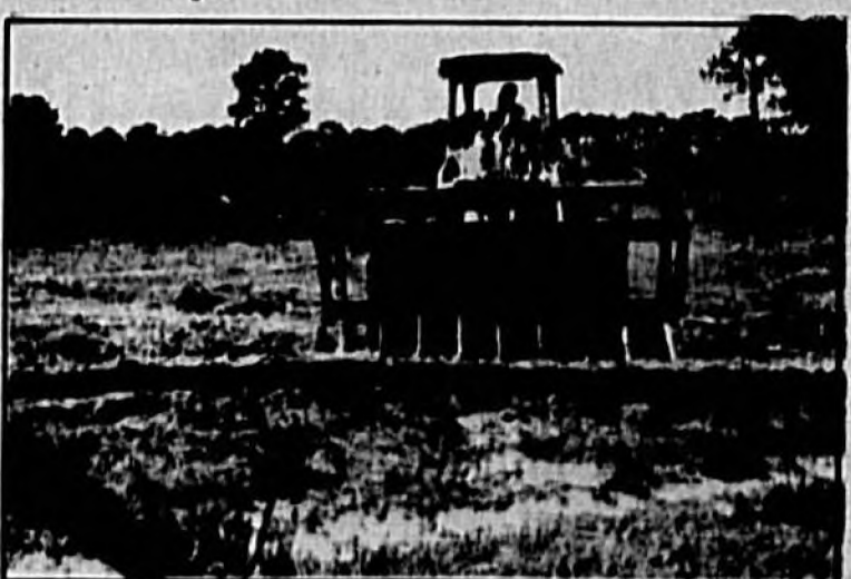
An equipment operator from Briar Corp. clears land for the new Sanford community swimming pool at Seminole County.
