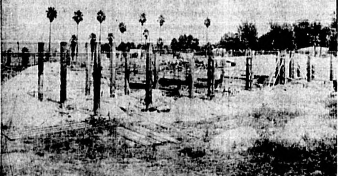
NEW COUNTY HOSPITAL—Primary work on the Seminole Memorial Hospital on E. Second St. is well under way. Work on the structure is being done by the Armstrong Construction Company, Palm Beach. It was contemplated by the hospital board of trustees to increase the capacity of the building to 100 beds, according to E. J. Thompson Sr., architect, but the plan was abandoned as not being feasible, and the structure will have a 75-bed capacity as originally planned. The hospital will have three floors and will be finished approximately in June. (Staff Photo)
