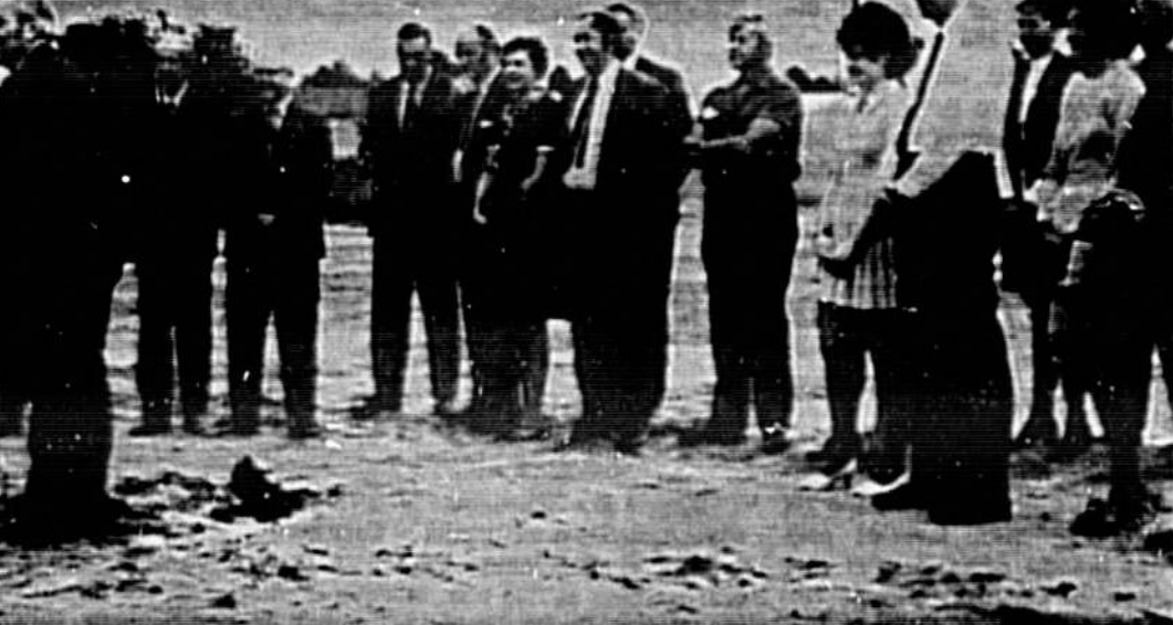
MAYOR LAWRENCE SWOFFORD and Vice Mayor Helen Keyser broke ground to begin construction of Altamonte Springs' new $220,000 civic center on a 20-acre tract south of SR 436. Attending the ceremonies were city officials, department heads and employees. Mayors Granville Brown, Curtis Blow and Kenneth Brown and Councilmen William Klossy of North Orlando, Casselberry and Longwood, respectively. Also present were Russ Hulbert of Winter Park Telephone Company, Ron Smith of Florida Power Corp., George Foster, Barnett Bank of Seminole County N.A. and James Cooper of First Federal Savings and Loan, Altamonte General Contractor for the facility expected to be completed before Labor Day is Sorenson and Fletcher and architect is Robert Webb.
