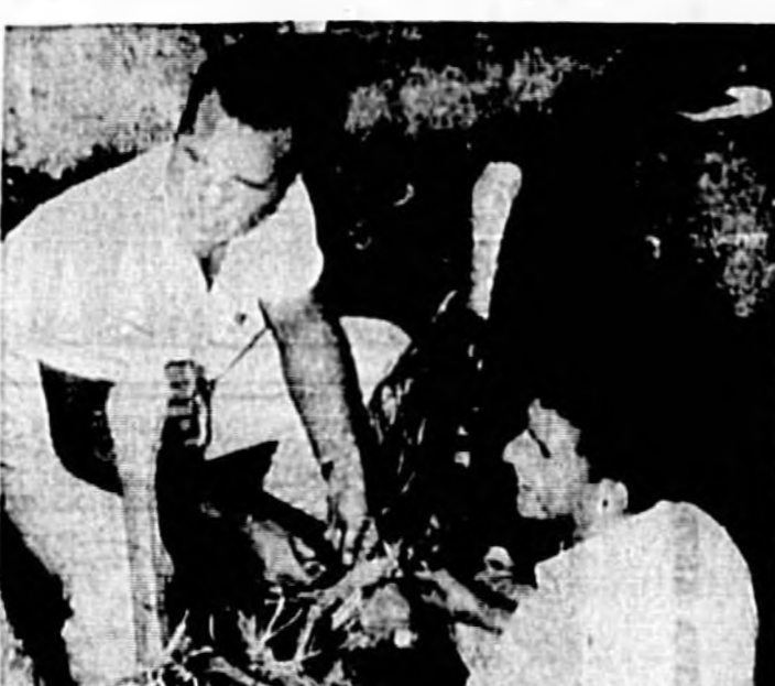
SPlicing CAbles IN THE PIt —Hundreds of tiny wires are joined together by E. C. Davitt (left) and David Van Ness, Southern Bell splicing crew. The finished cable will bring telephones to hundreds of Sanford homes. (Bergstrom Photo)
