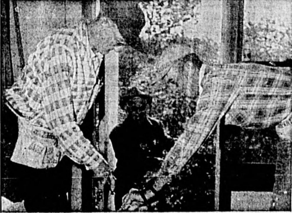
THE NEW FIRE ESCAPE DOOR is being put in place at the Sarepta Rest Home by Johnny Lee, Thurman Smith and Edgar Osborne.
