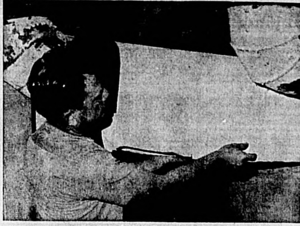
LEROY "RED" GROOVER of Wall Plumbing assists other workmen in installing sheeting over furnace pipes at the Sarepta Rest Home.
