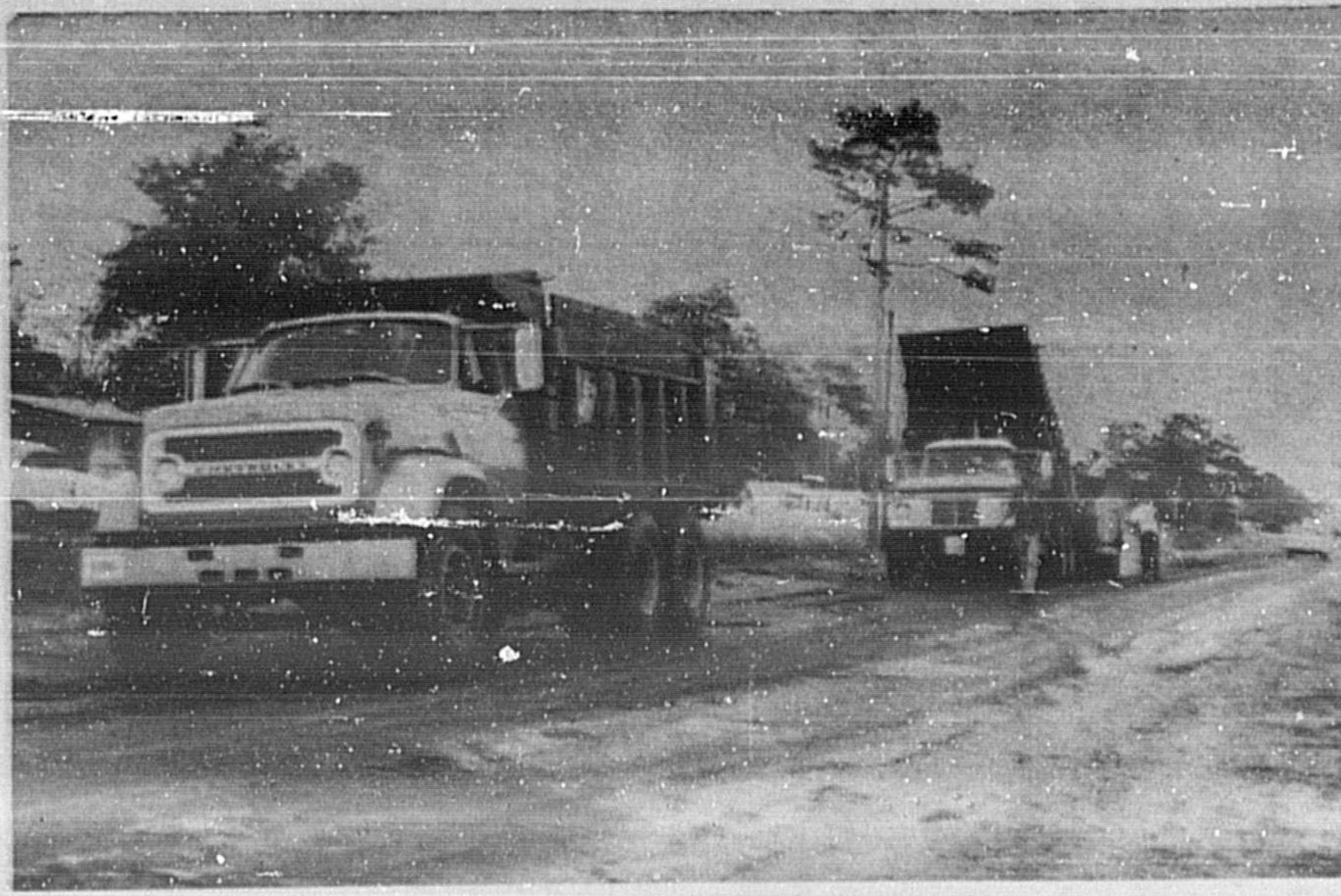
PAVING IS UNDERWAY on a new access road leading to SH 436 from the beautiful Seminole Turf Club in Casselberry. The thoroughbred racing schedule at the club gets underway April 20 for 90 straight nights of racing.
