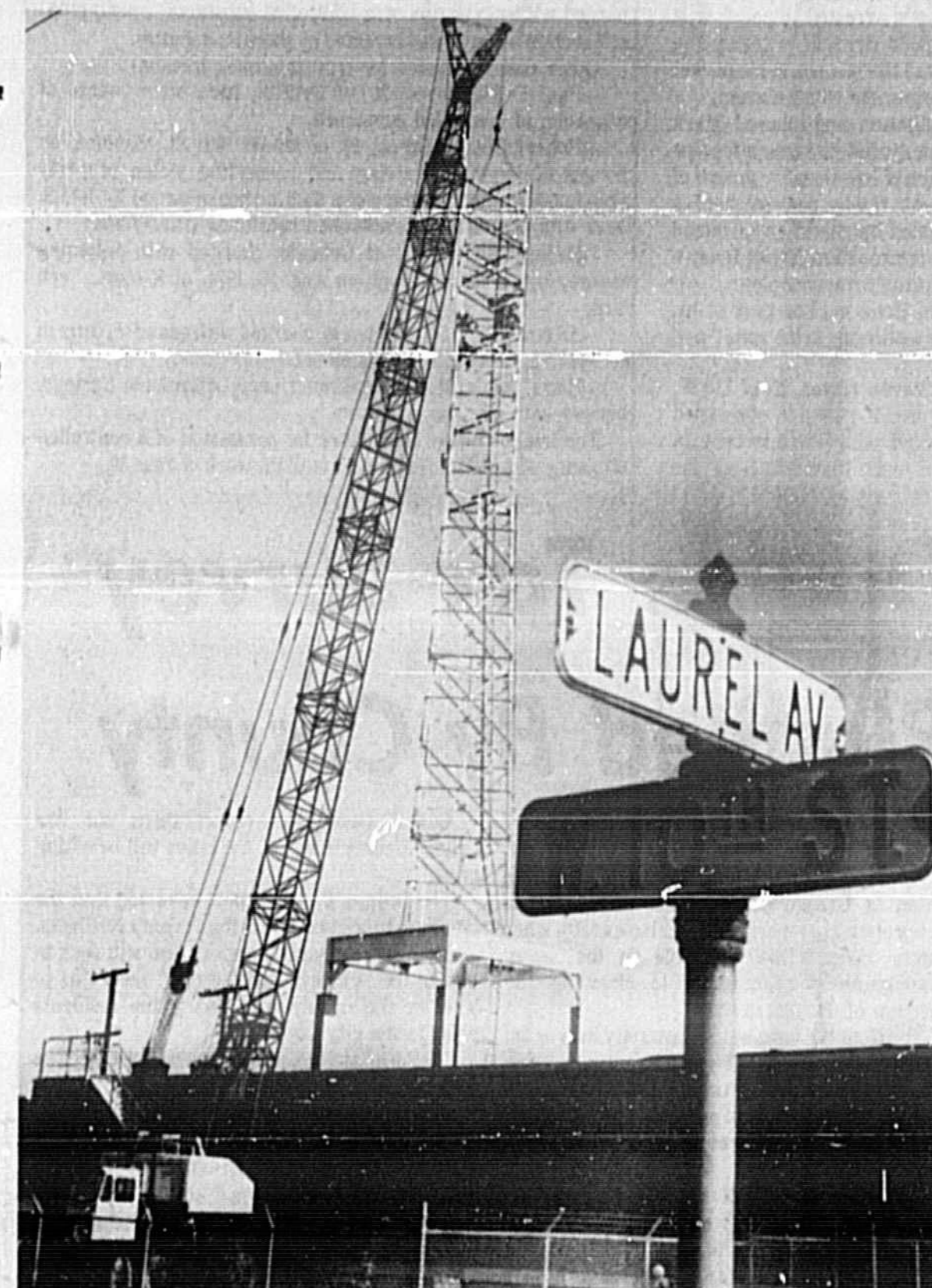
PHONE TOWER GOING UP. Work is moving along on Southern Bell's 125-foot microwave telephone tower...
