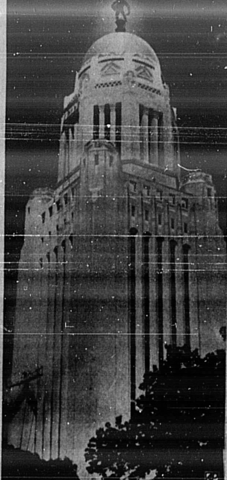
COMES CLEAN — Tower of state capitol building in Lincoln, Neb., gets a cleaning. From this angle, tower dwarfs man on scaffold who works on stone. Statue atop tower is called the sower.
