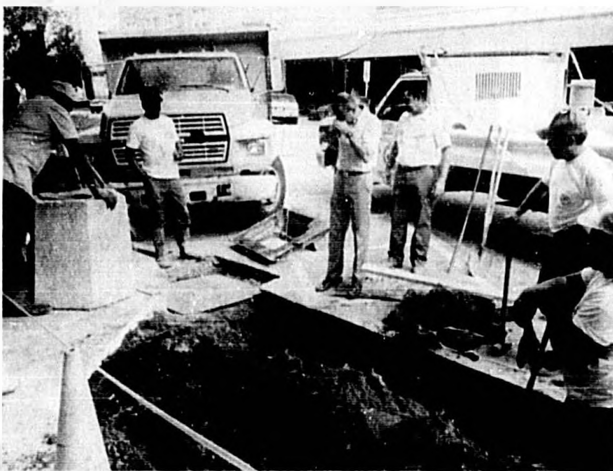
A bit of history was dug up yesterday. City workers installing new wheelchair ramps in the 100 block of E. First Street, uncovered remnants of old storm drains. "We call them box-culverts," said Street Maintenance super-
