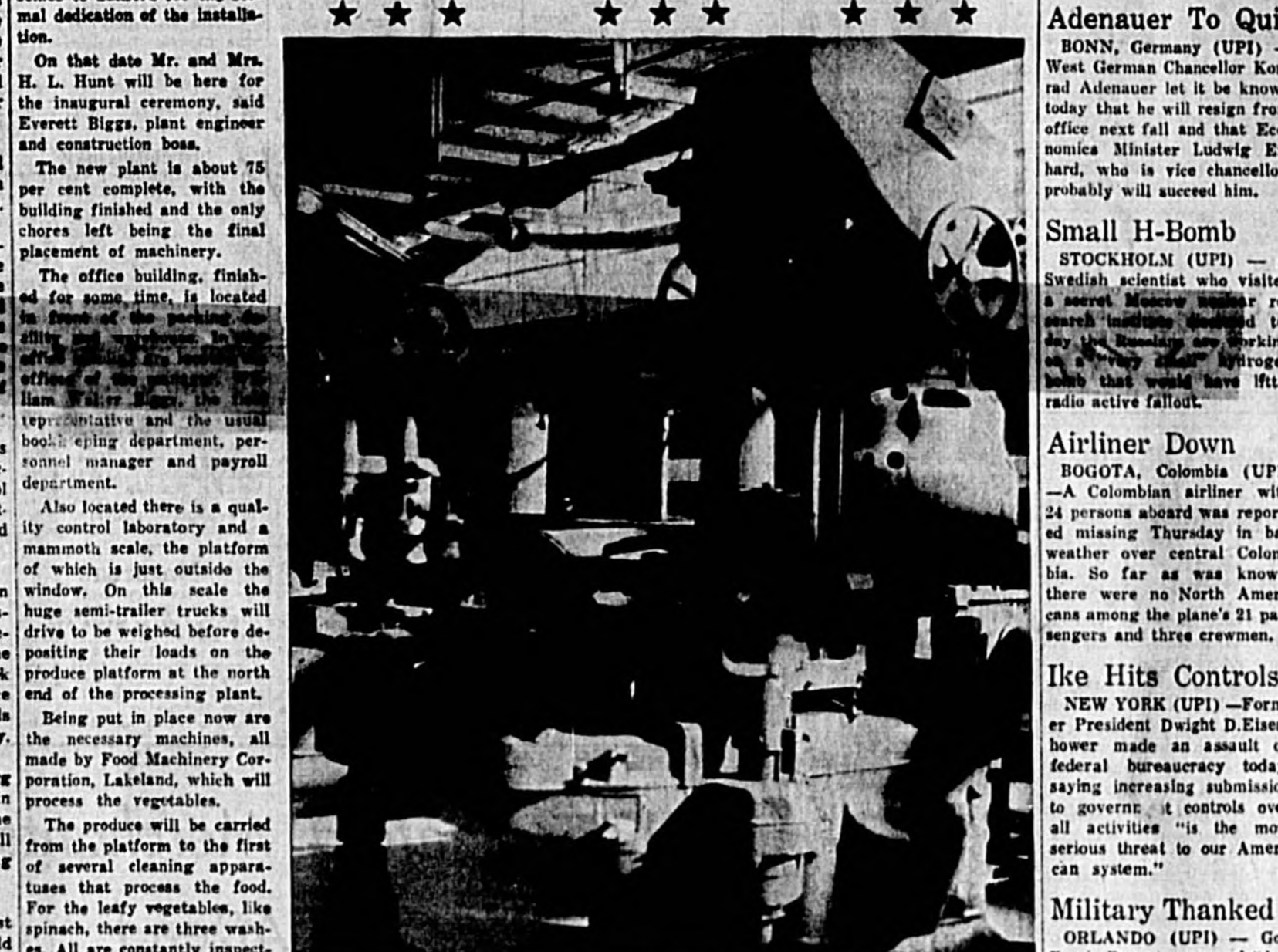
Part Of Battery Of Canning Machines Installed
