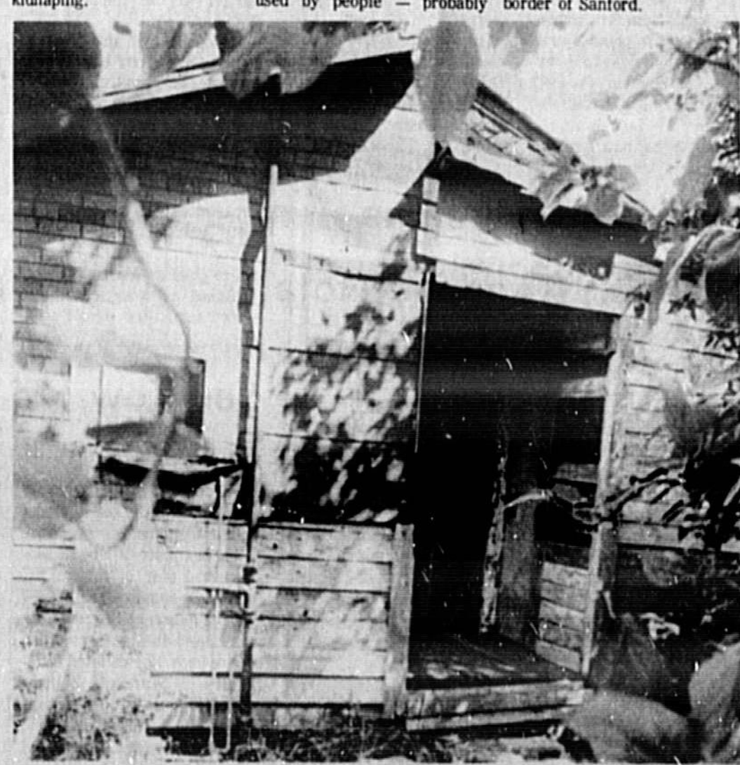
REAR SEALS BROKEN BY INTRUDER... Day after investigators searched house
