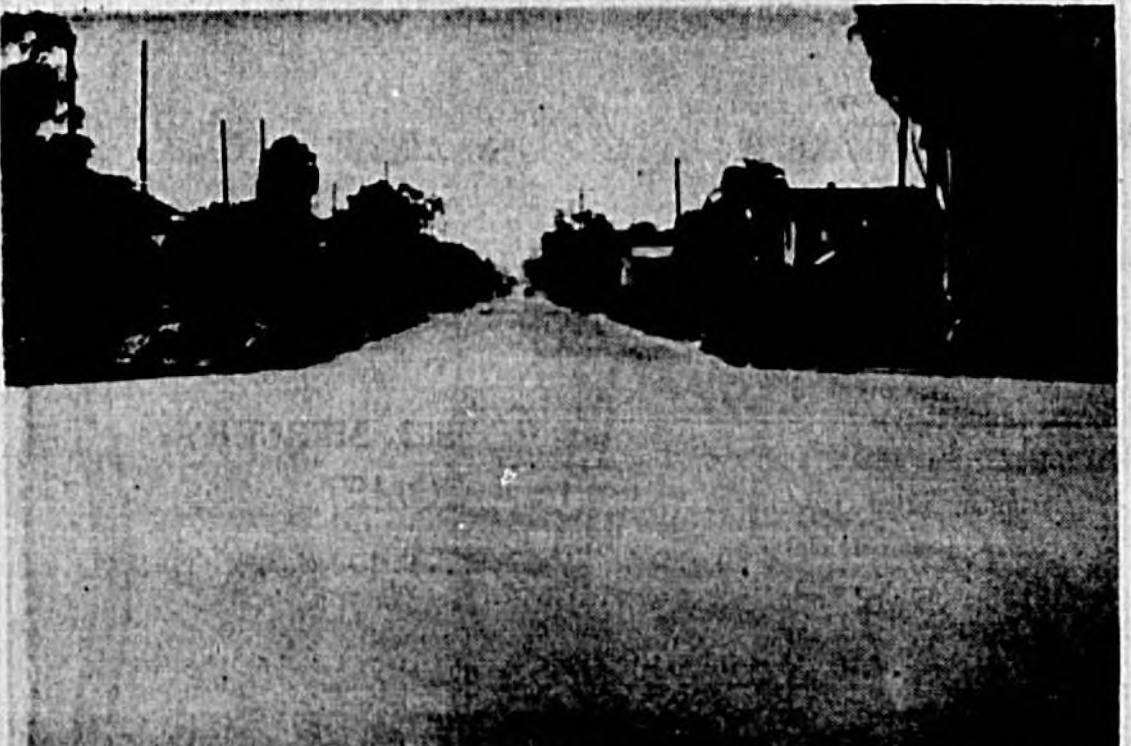
WEST — Widening First St. From French Ave. to Inter-State Hwy. Exit at Lake Monroe.
