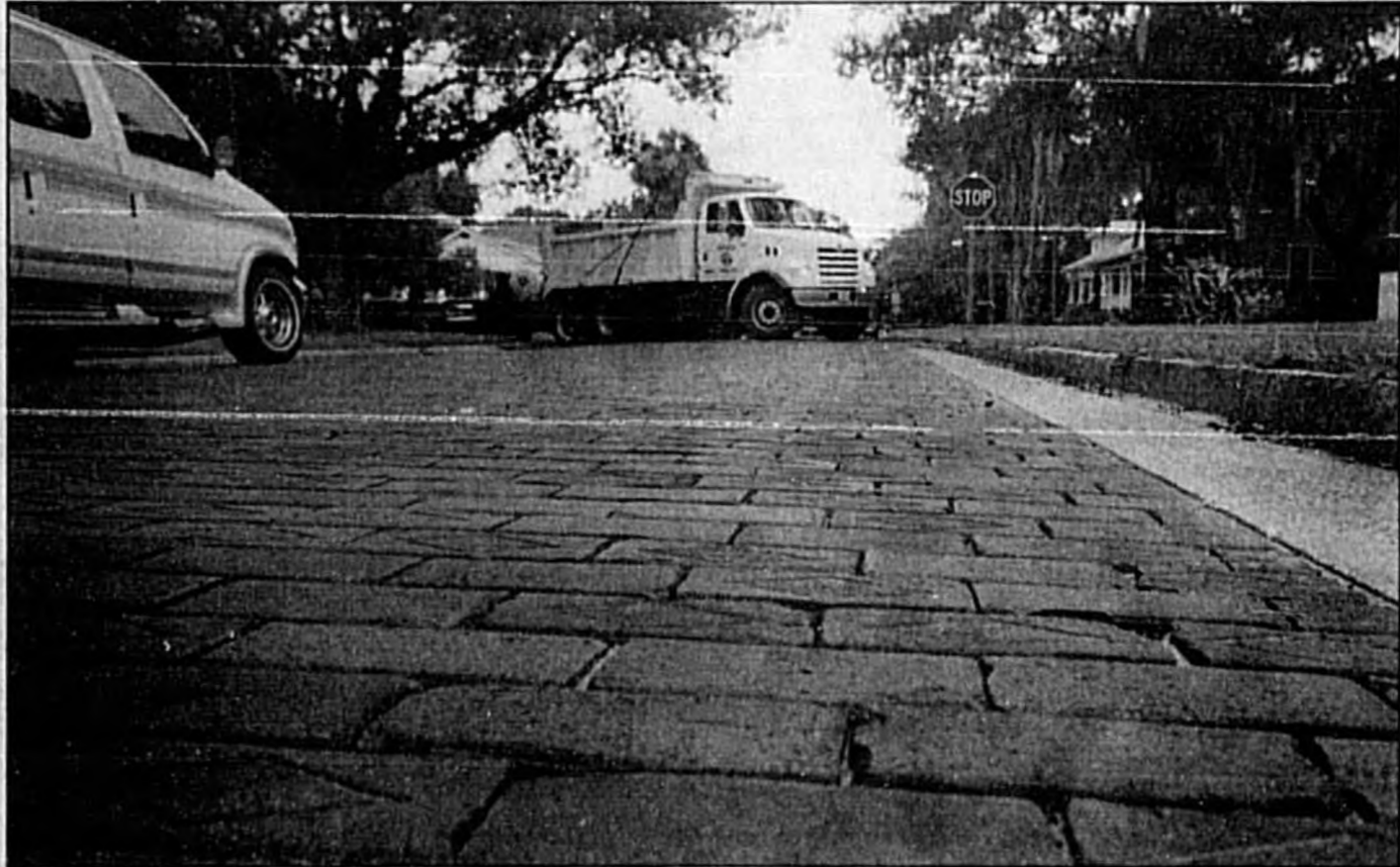
The city of Sanford is exploring ways to restore about 6 miles of streets to their original brick layout. The bricks have been paved over with asphalt. Pavement Savers Inc. of Cocoa demonstrated a process that heats the asphalt so it can be removed without damaging the bricks.
