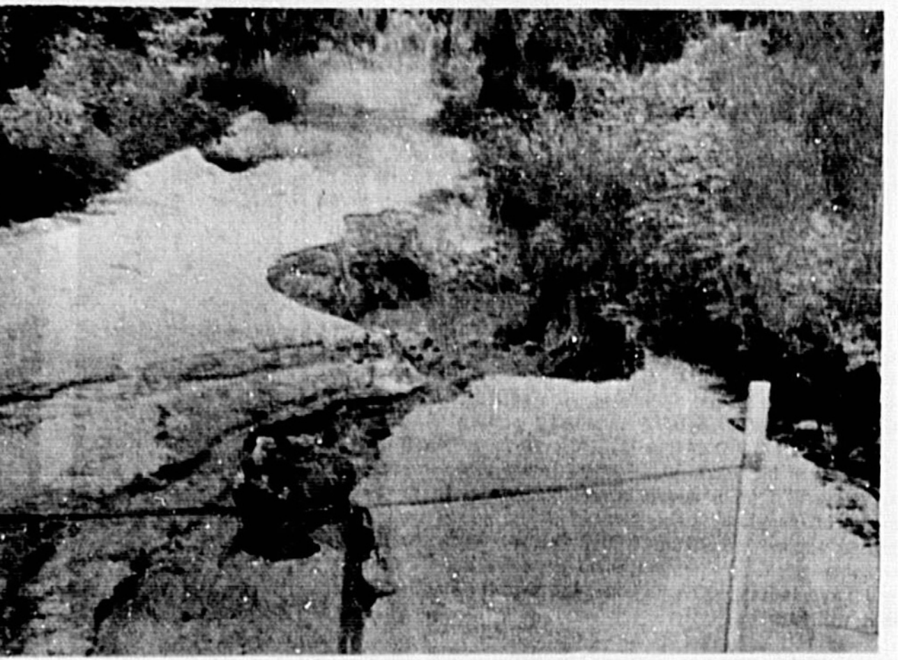
AND AFTER THE RAINS drained, it caused extensive damage like this area on County Road, North of Orange Boulevard.
