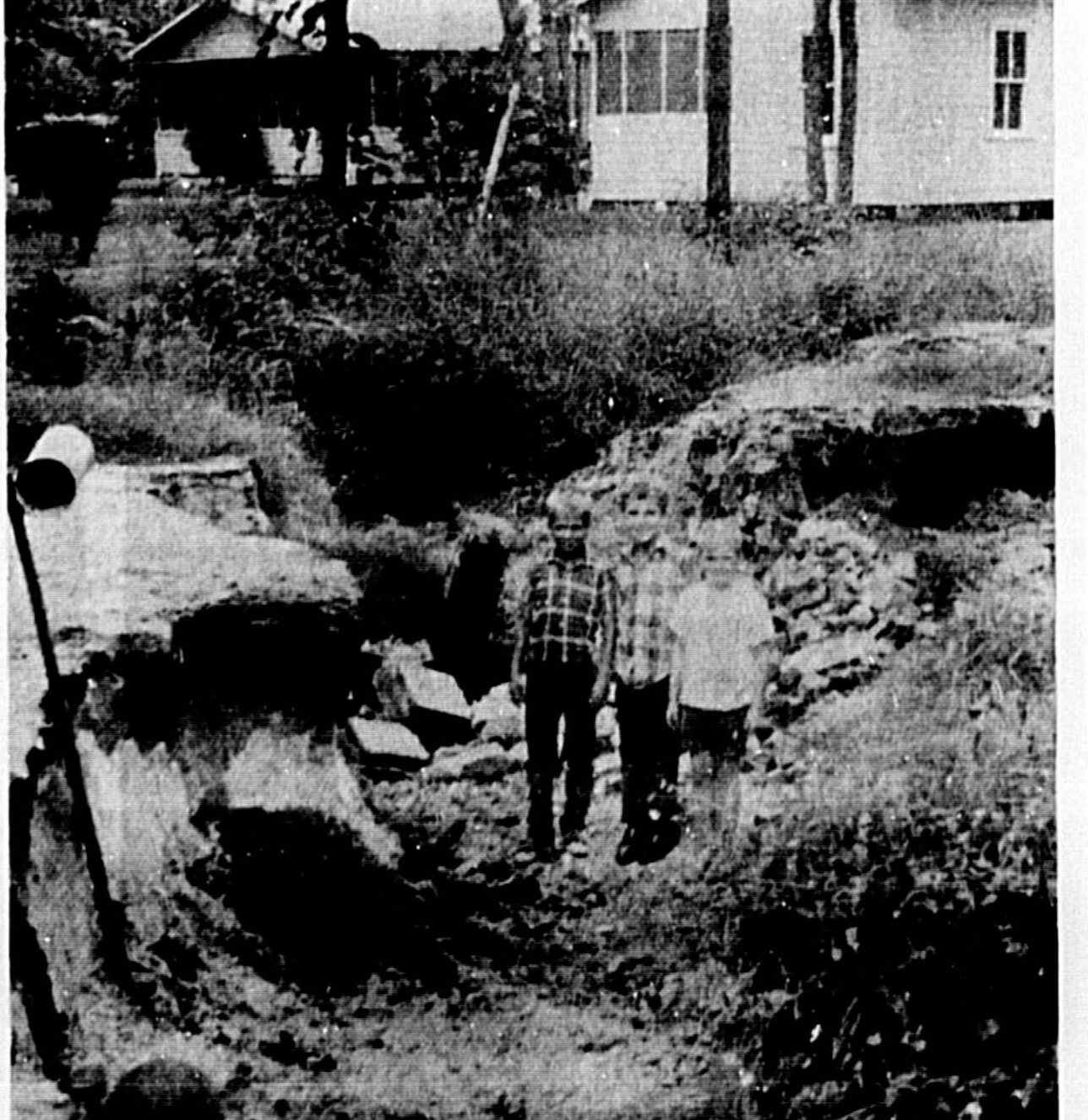
INSTEAD of the water flowing through the small culverts, debris clog the entrance to the pipe, forcing the water to overflow causing this major washout in the Lake Monroe area, adjacent to I-4. (Staff Photos by Bill Vincent).
