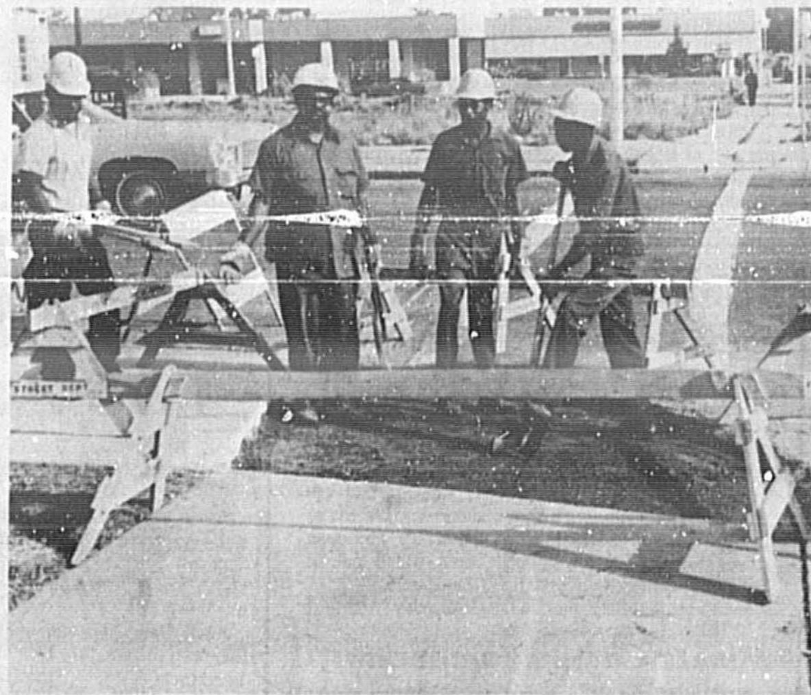
City construction crews today were busy installing wheel chair ramps at First Street and Sanford Avenue. Ramps and special parking spaces for people confined to wheelchairs are being built on Sanford's downtown streets. (Herald Photo by Bill Vincent)
