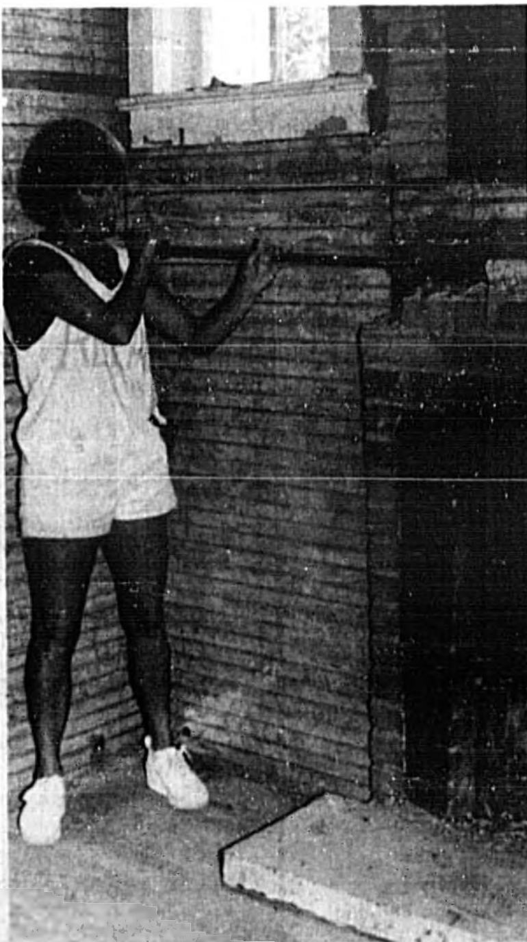
Using a crowbar, Thanna Kulash removes old bricks from a fireplace in one of the Sanford homes she is restoring.
