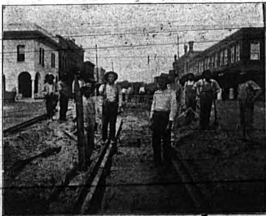
The above photo was taken while the workmen were busy laying the rails for Sanford's new street railway. The line will extend for five miles east to Cameron City and five miles west to Monroe, thus giving Sanford a belt line. A fine amusement park will be constructed along the line of the new railway.
