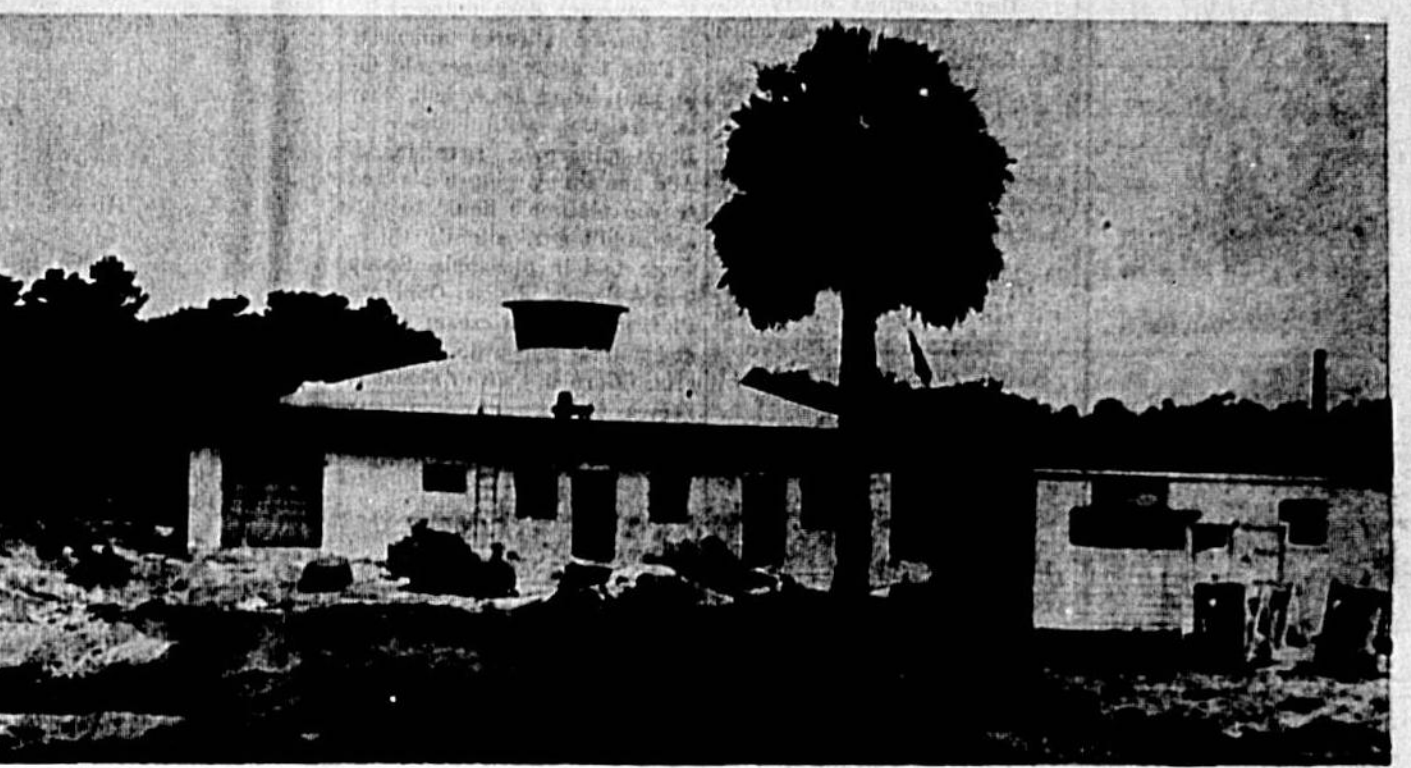
WELLS, water tank and maintenance facilities for the new Oviedo water system are way ahead of schedule. The new facilities are located one mile south of the center of the town. All the mains have been laid and fire hydrants installed. Workmen are now busy installing water meters. (Herald Photo)
