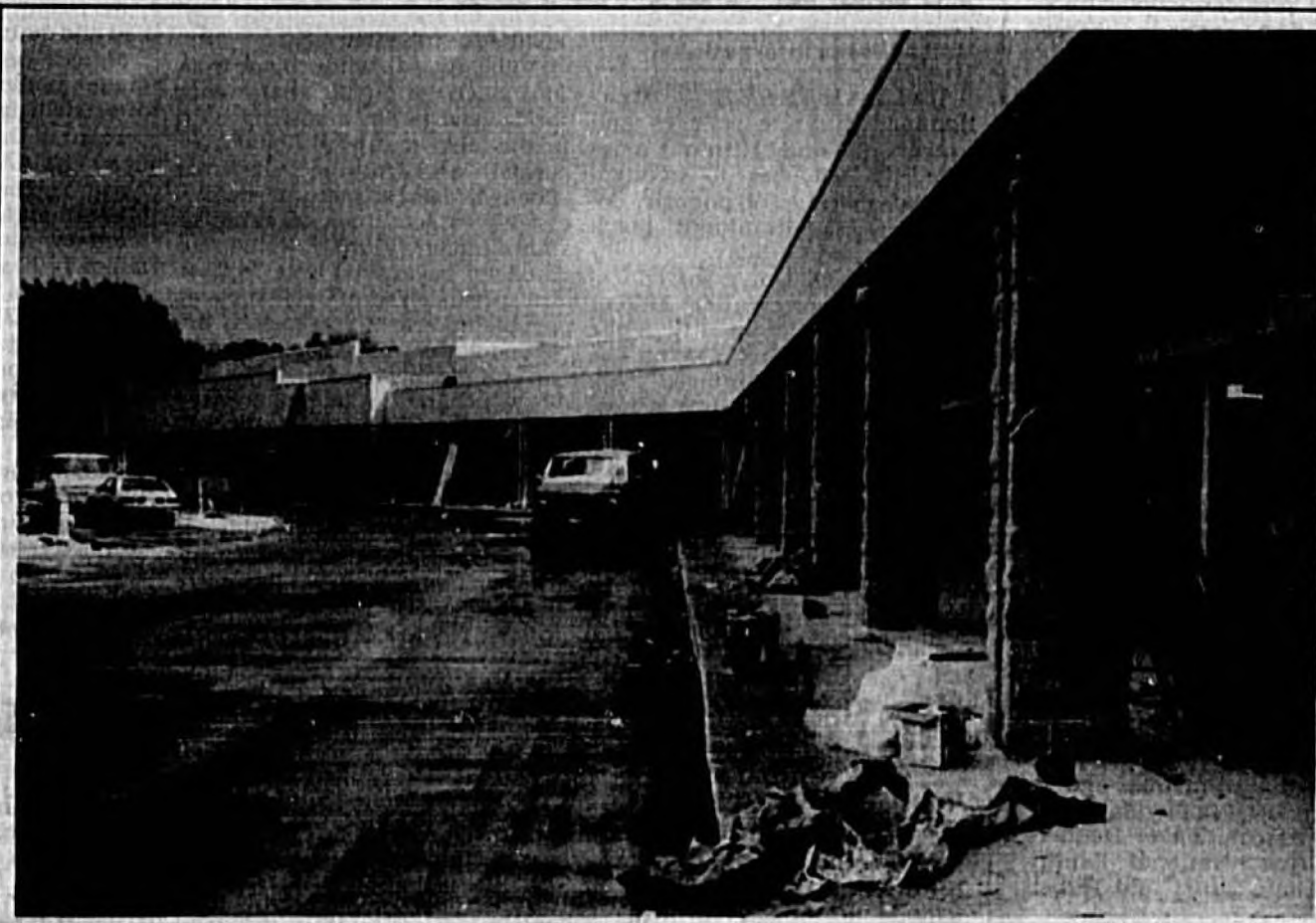
Work continues on The Oaks Shopping Center, now a topic of controversy.
