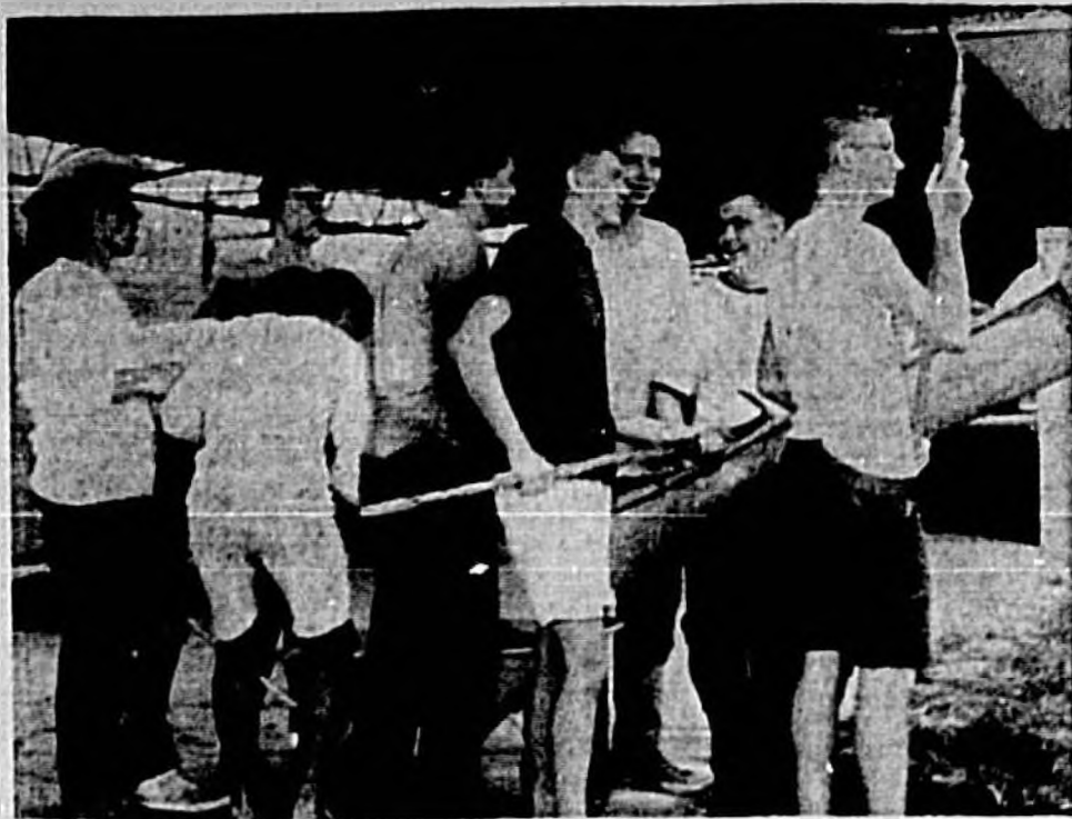
KEY CLUB members at Seminole High School spent Friday afternoon laying a 65-foot sidewalk from the school library to the street. The boys, sponsored by the Kiwanis Club, also bore the cost of the materials from funds they derived from various projects. (Herald Photo)
