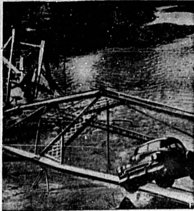
SHORTLY BEFORE it toppled into Loyolhanna Creek, an auto hangs precariously from the beam of a collapsed bridge at Salisbury, Pa. The driver, Ed Fennell, of Fenneltown, Pa., escaped with minor injuries when heavy traffic weakened span causing it to give way.
