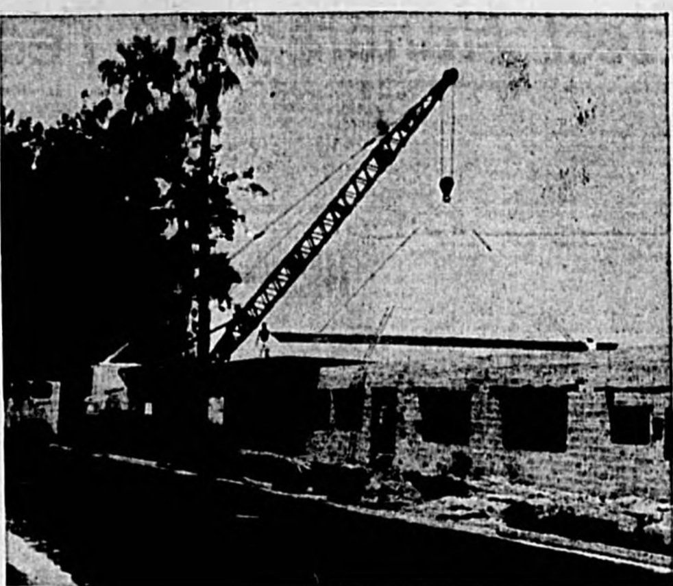
THE ROOF GOES ON the cafeteria building which is now under construction at Sanford Junior High School. Workmen are busy with this and the construction of a band and music room, and a library. The buildings are expected to be completed this year but no opening date has been set.
