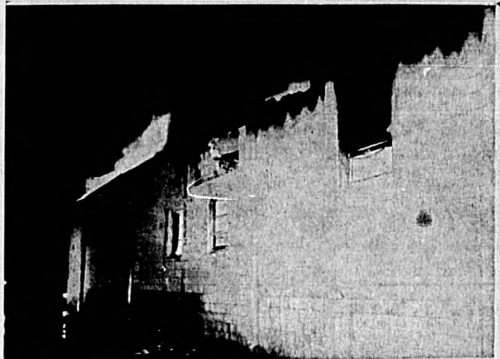
... believed to have started shortly after midnight this morning. Cause of the fire is unknown but it is believed it was faulty wiring.
