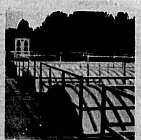
But odors have been reduced, plant officials say, by these caps which were placed atop the conditioning ponds at the plant.
