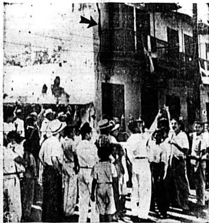
A STREET CROWD points to large crack (arrow) in a building in Ciudad Trujillo, Dominican Republic, after an earthquake and a tidal wave caused heavy damage in the Caribbean republic. Neighboring islands and areas on the northern coast of South America were also damaged by the earthquake and the high waves. (International Soundphoto)
