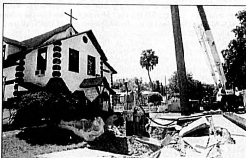
A stormwater drain collapsed in front of Victory Temple of Praise Church on Pine Avenue. The collapsed caused moderate damage to the church.
