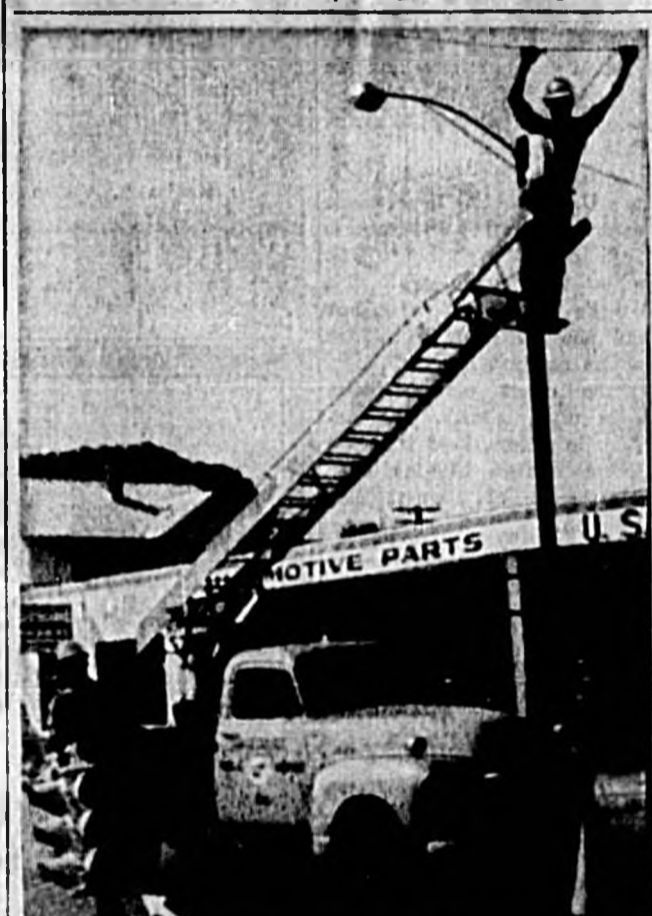
AND AWAY WE GO... City work crews today removed the traffic light at Second and Park as the first step in the downtown improvement plan making Third St. a thru street. The light will be placed at Third and Park. (Herald Photo)
