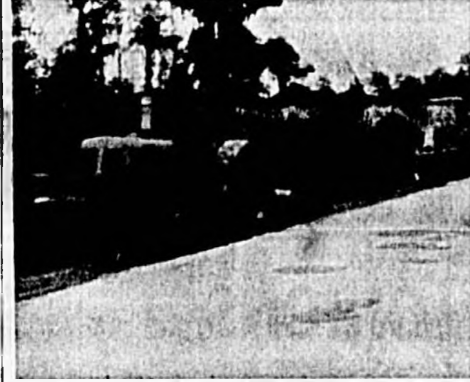
WORK IS progressing on widening Seminole Blvd. to the Seminole Raceway. The project, which calls for widening of six feet, is expected
