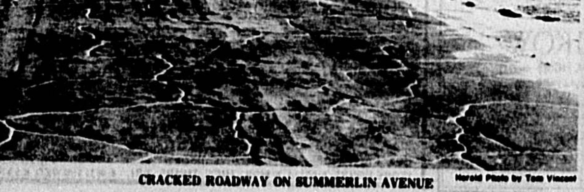
CRACKED ROADWAY ON SUMMERLIN AVENUE
