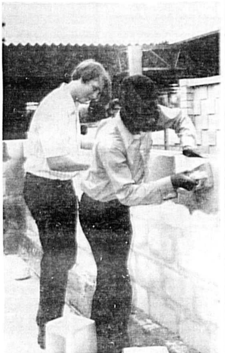
PRACTICAL experience is gained by Ron Nelson (right) and Robert Hansen of Angel Mender masonry II class at Seminole High School as they construct a storage building.
