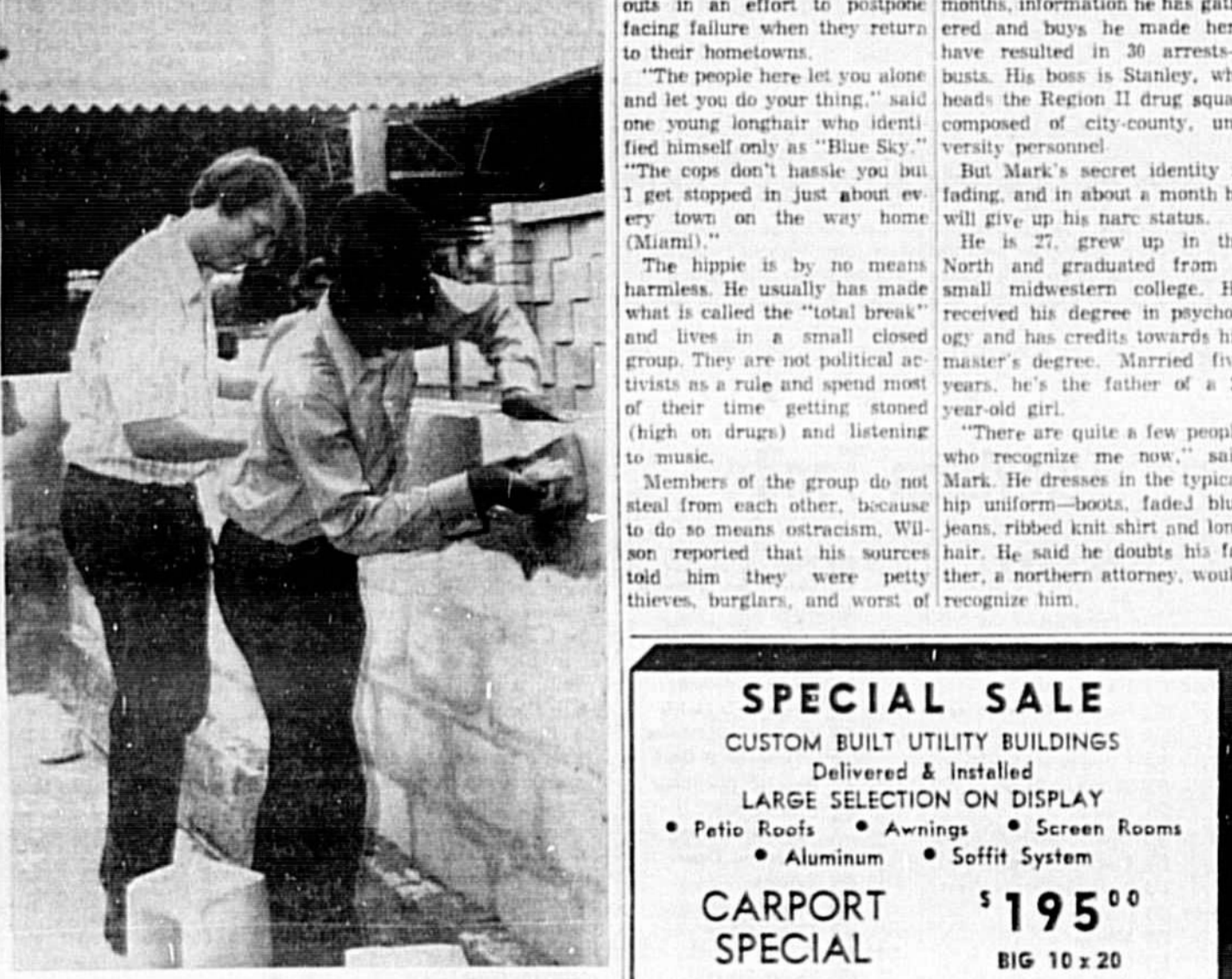
PRACTICAL experience is gained by Ron Nelson (right) and Robert Hansen of Angel Mendez' masonry II class at Seminole High School as they construct a storage building.
