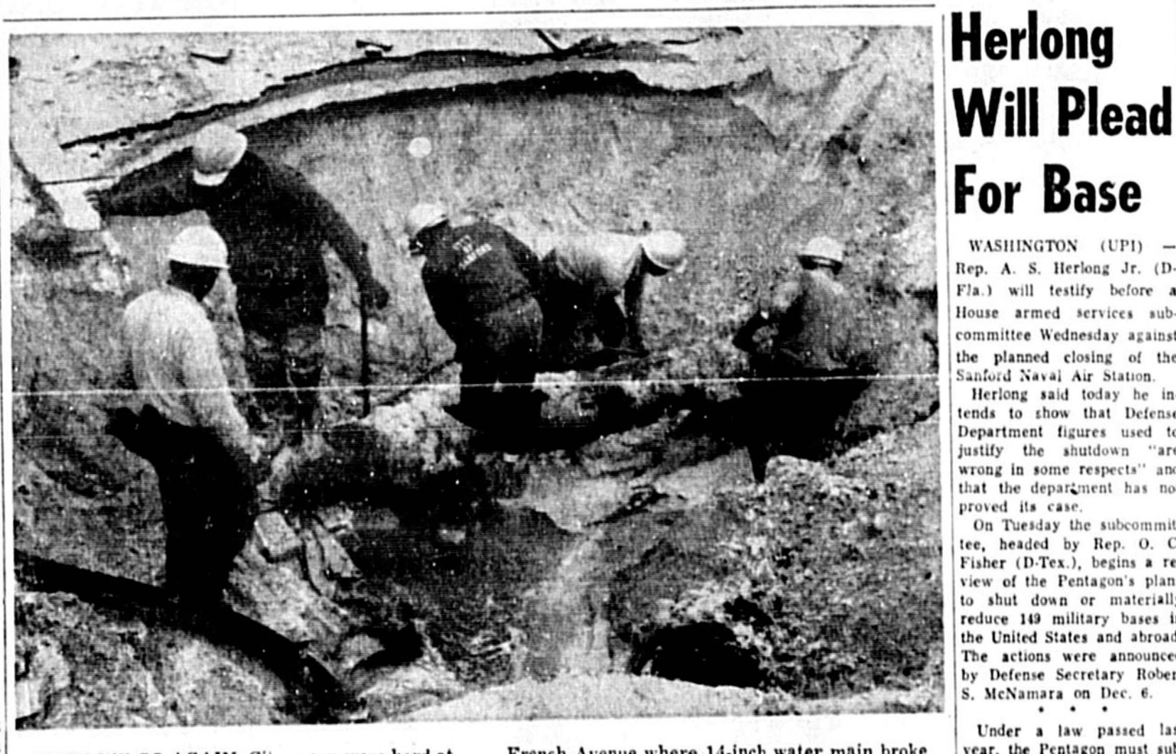
HERE WE GO AGAIN. City crews were hard at work today repairing damages to another burst water line - this one in the 1800 block of French Avenue where 14-inch water main broke Thursday night.
