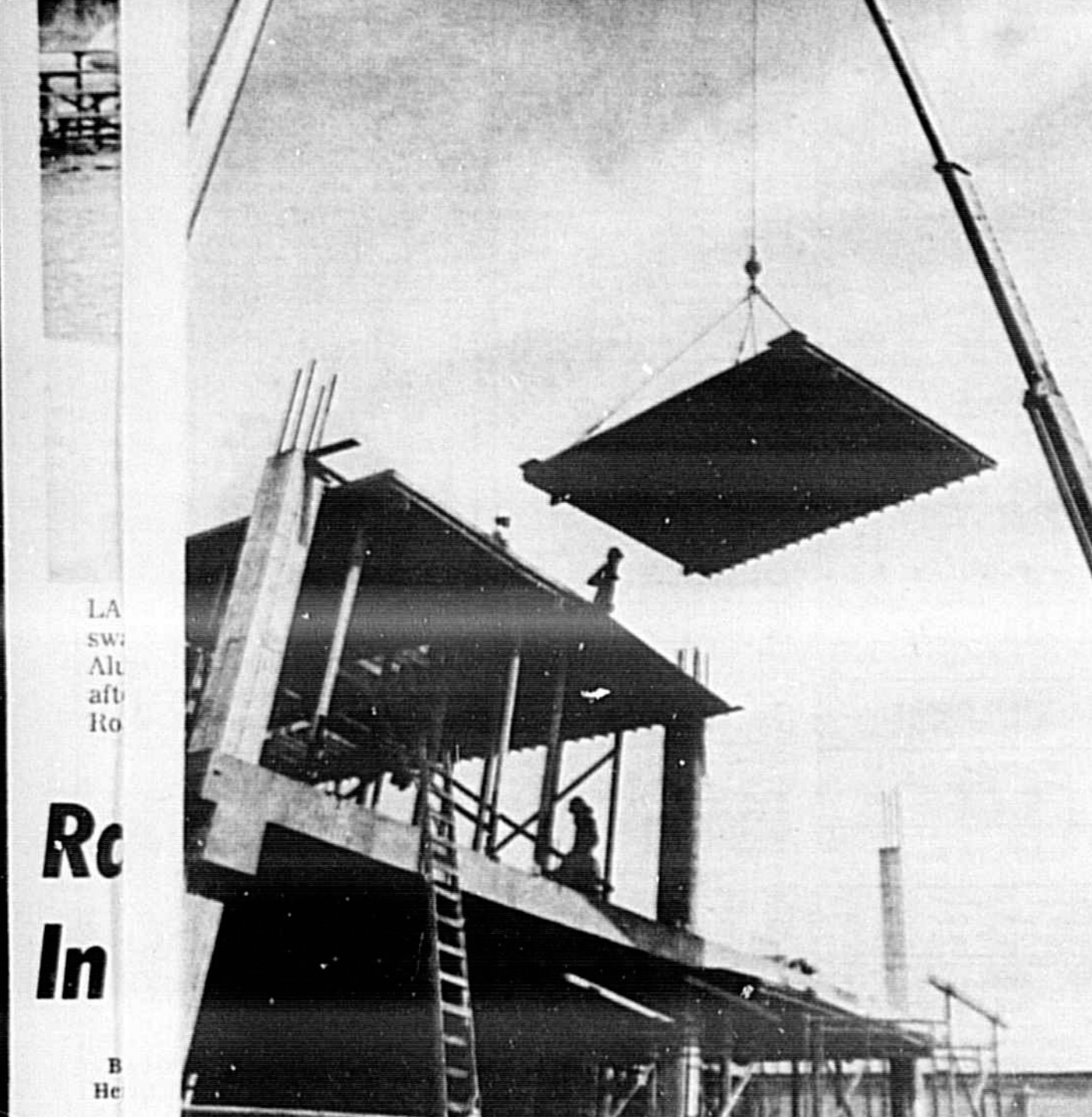
WORKERS ARE silhouetted as construction crane lifts portion of large form into place prior to pouring of third concrete floor at First Federal Savings and Loan Association of Seminole's new four-story office building addition on West First Street, Sanford. The new building is scheduled now for completion in November by general contractor Williams Development Co. of Orlando. Another portion of the institution's expansion program, $125,000 in additional drive-in teller facilities to the west of the main building, were recently opened to customers.
