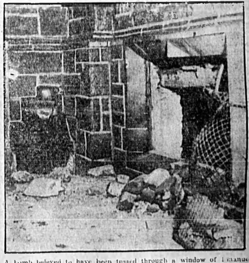
A bomb believed to have been tossed through a window of Emanuel Presbyterian church, Philadelphia, wrecked the basement, broke all the windows and threw the neighborhood into a turmoil of excitement. This photo shows how a section of the lower wall was ripped out by the blast.
