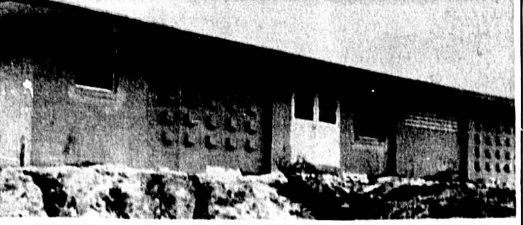
WORK is progressing on the Eastbrook Pool Association project in Eastbrook. The concrete bathhouse (top) is scheduled for completion by the end of the week and will cost $14,789. It contains lobby, snackbar, shower and locker rooms. The Junior Olympic Pool (bottom) being built at a cost of $37,147 is expected to open sometime in September. Site work, costing $6,425, also has been started, beginning with grading for road, picnic area, parking space and tennis courts.
