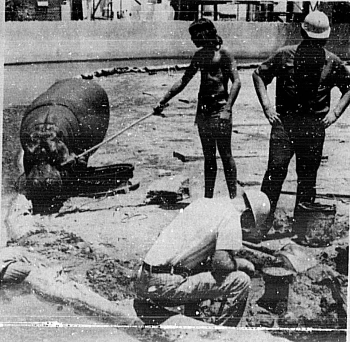
SINKHOLE AT ZOO A huge sinkhole opened up at the Central Florida Zoo, temporarily displacing a hippopotamus, watching warily at far left. City workers Jim McCracken, sitting, Robert Davenport, unseen in sinkhole, and Ben Howard work on the problem while Jim Mauldin of the zoo keeps Pat Boy out of the way. (Herald Photo by Bill Vincent)
