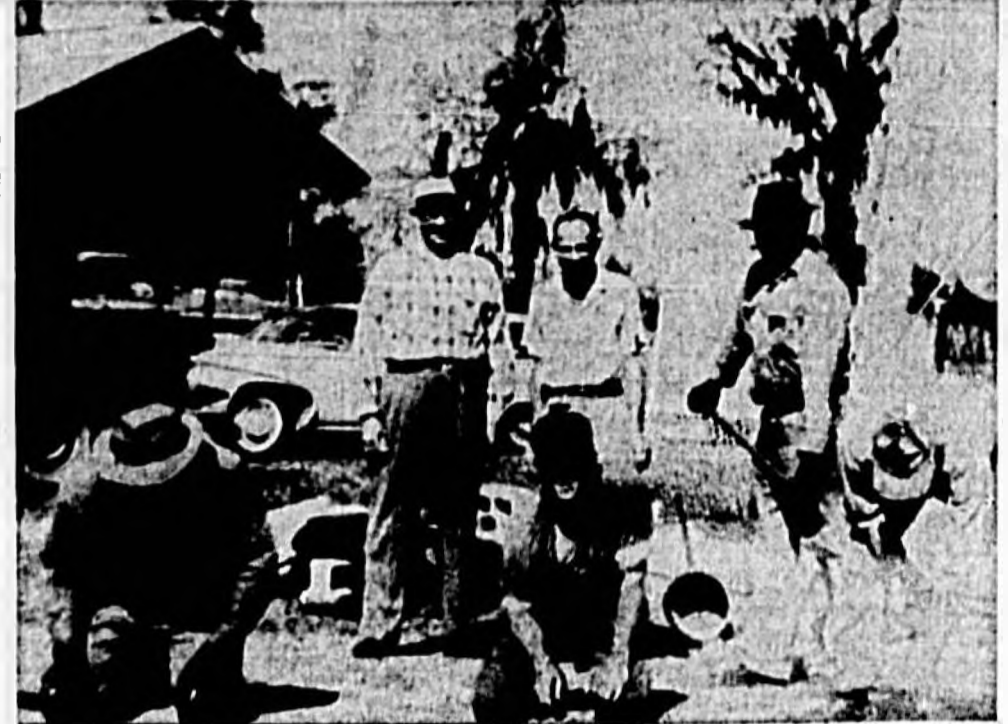
CASSELBERRY UTILITIES CO. crews finished off the foundation for a new 116,000 gallon prefabricated metal tank Monday morning to complete the initial step of a major improvement program for better water and service. Workmen Ed Simmons, Dallas Brown, Charlie Williams and Willie Harris, left to right, were supervised by Paul Bates, company superintendent, right back, and "Sidewalk Superintendent" Bill Tilford, left back. (Herald Photo)
