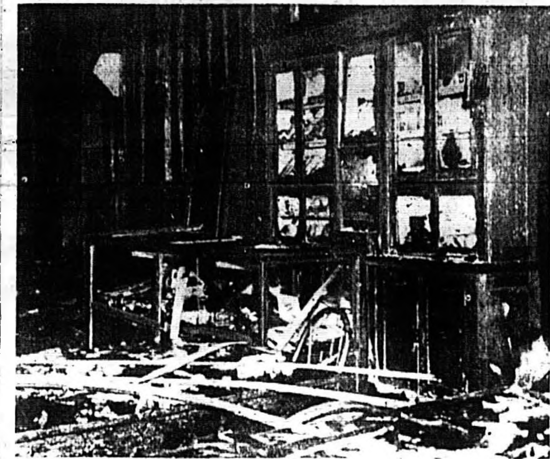
DEBRIS is scattered through the lobby of the old Canfield Hotel in Dunwoody, where fifteen persons lost their lives in a fire which started in the lobby and spread rapidly through the building and its six-story annex.
