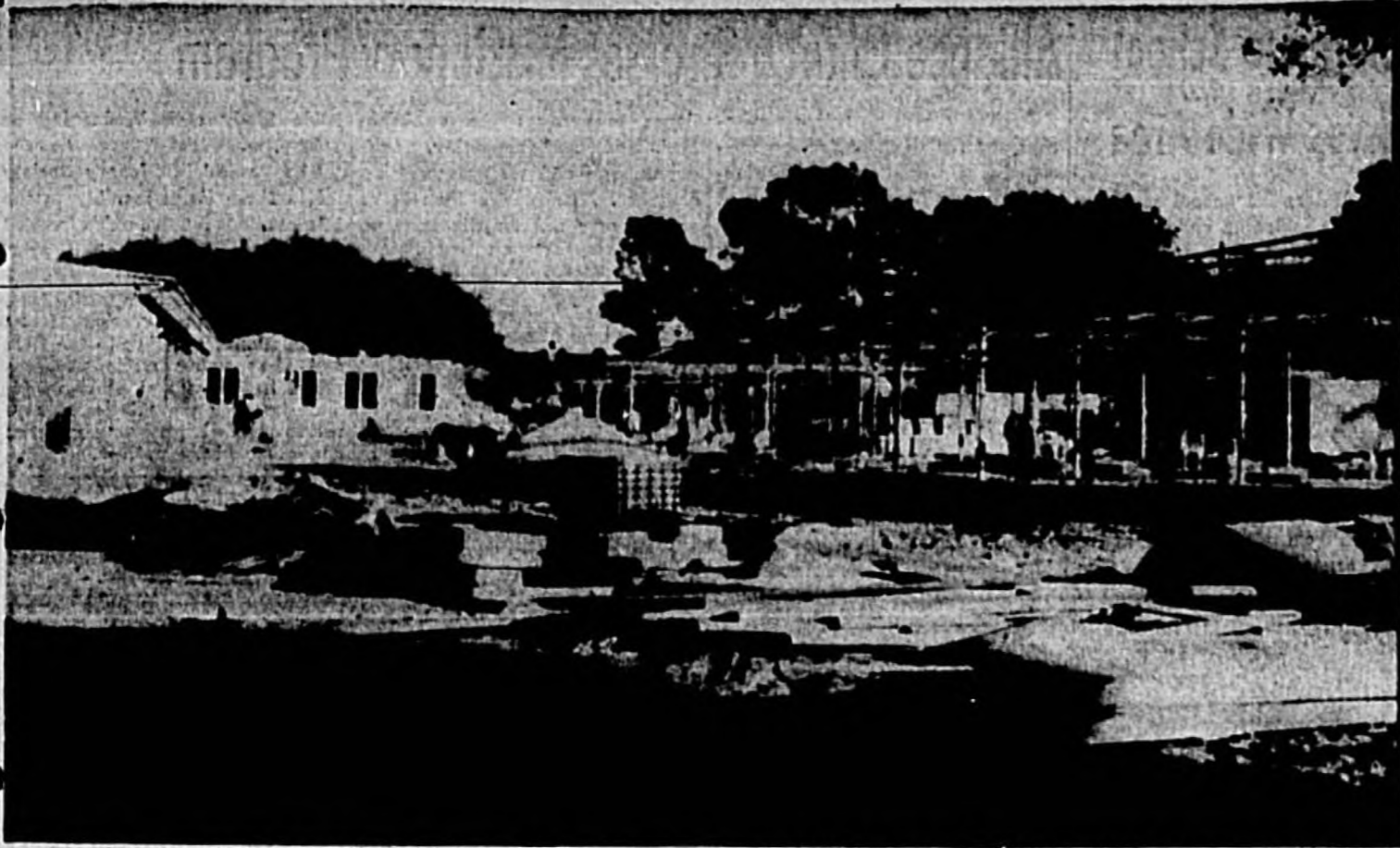
EACH SECTION OF SEMINOLE COUNTY produces scenes like this of school construction this year as the program is pushed to get added school rooms for
