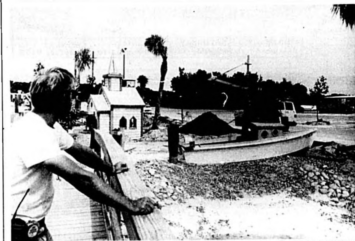
Danny Polley, supervisor of construction for the Fun World project, takes a look at the still unfinished portion of one of the park's miniature golf courses.
