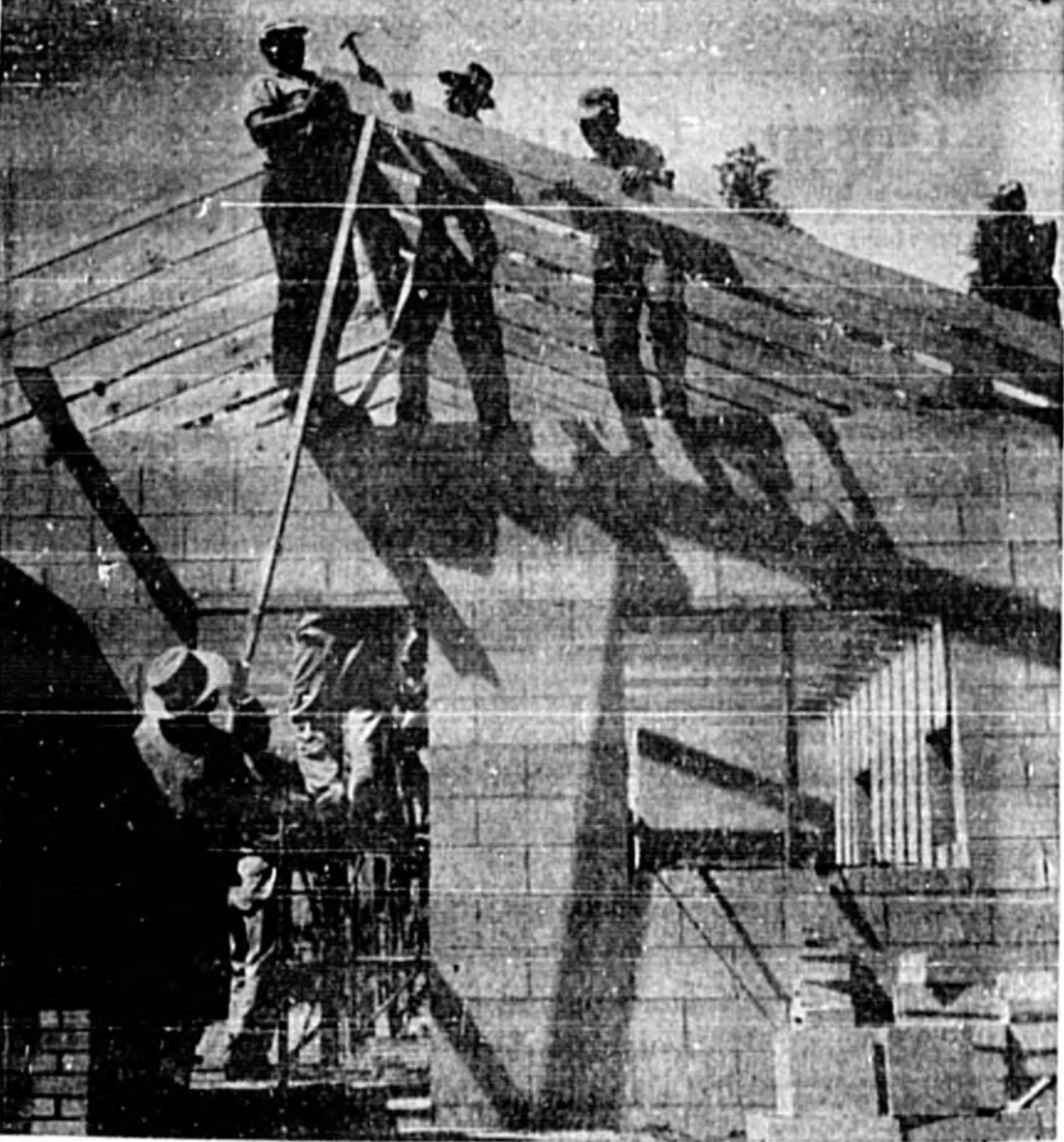
THE ROOF GOES ON the Oriedo American Legion Building Saturday afternoon. Shown putting the rafters in place are: A. B. Tredford (on the ground) Jim Parlin, Frank Wheeler Jr., T. L. Hango and George Means (top above). The building is expected to be ready for dedication on June 1. (Photo by Bergstrom)
