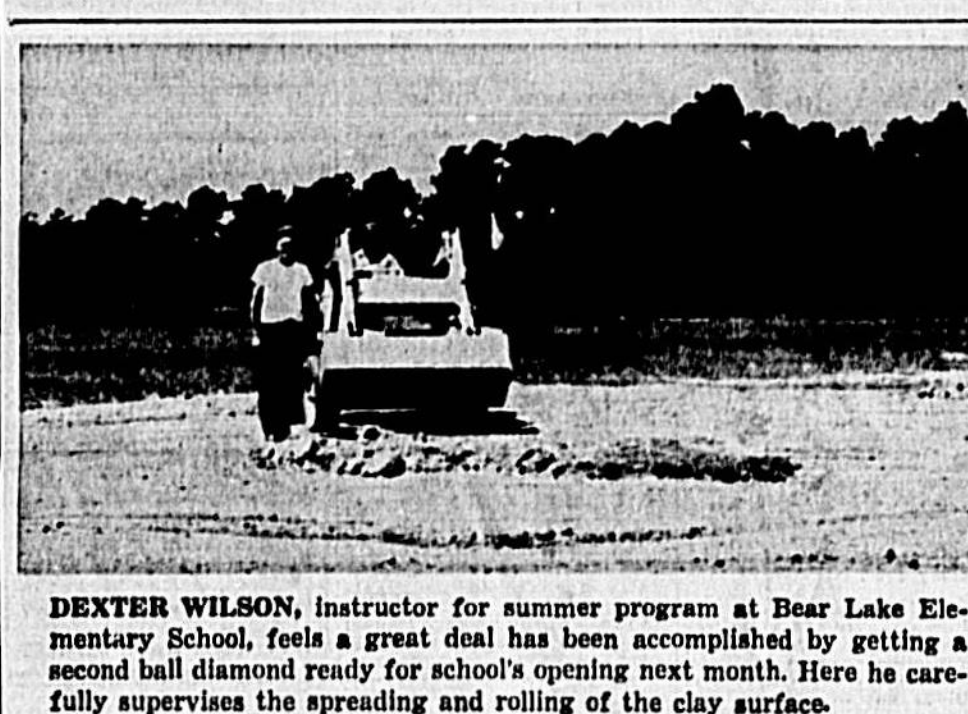
DEXTER WILSON, instructor for summer program at Bear Lake Elementary School, feels a great deal has been accomplished by getting a second ball diamond ready for school's opening next term. Here he carefully supervises the spreading and rolling of the clay surface.
